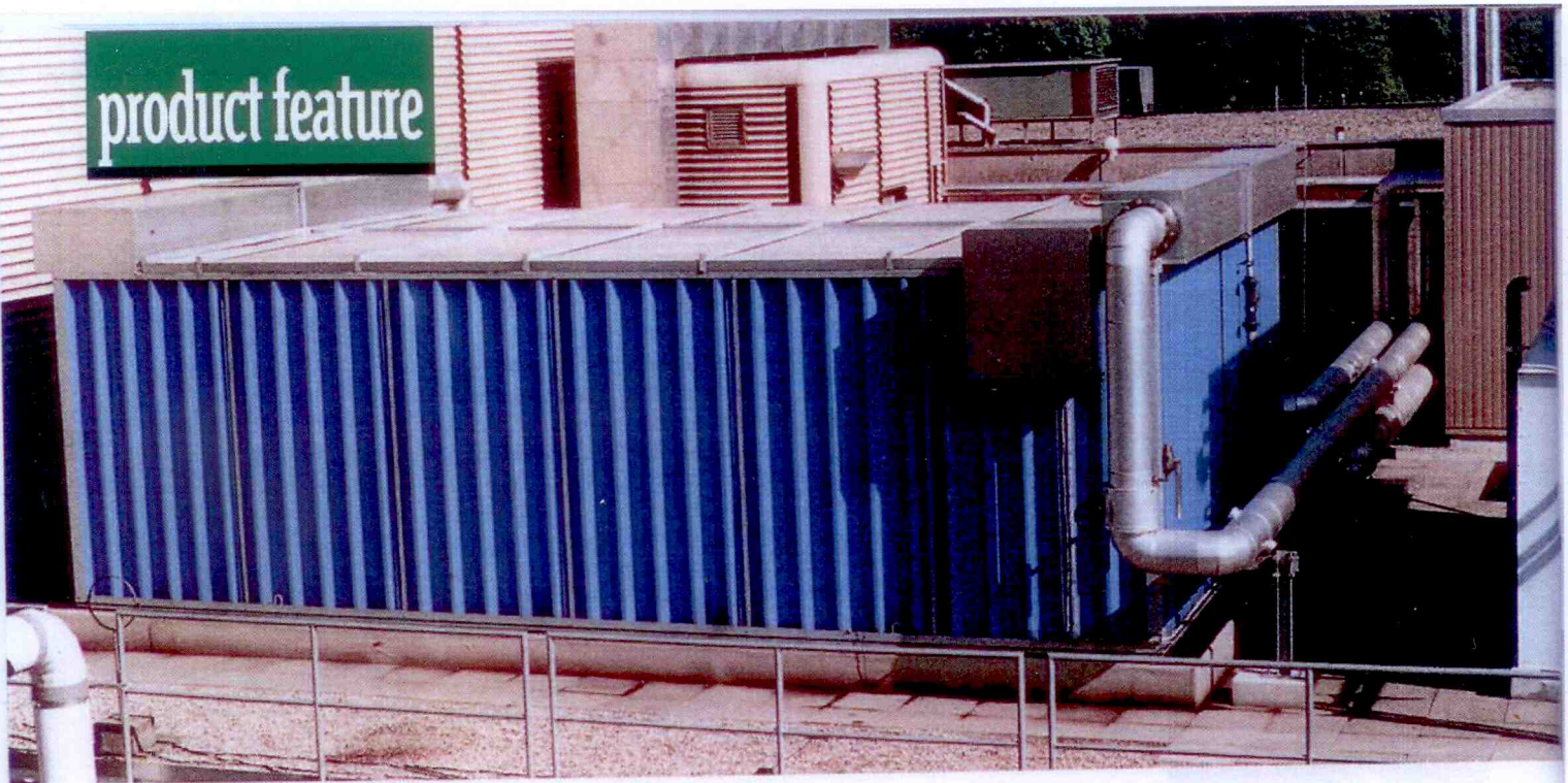
An ice thermal storage system | Imec Electromechanical Engineering
