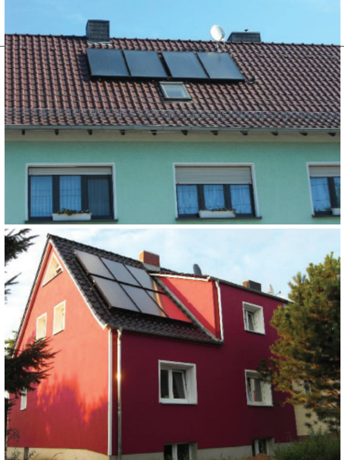
Baymak-BDR Thermea Group Solar Water Heater Installations in Germany.
