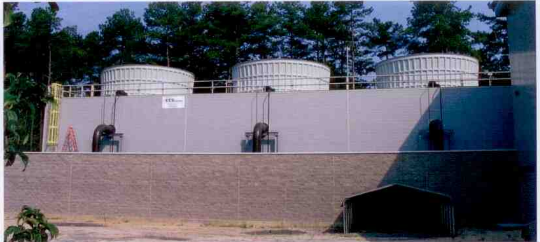
Some once-through cooling systems in the region have reached a flow rate six times that of the River Thames in London.
