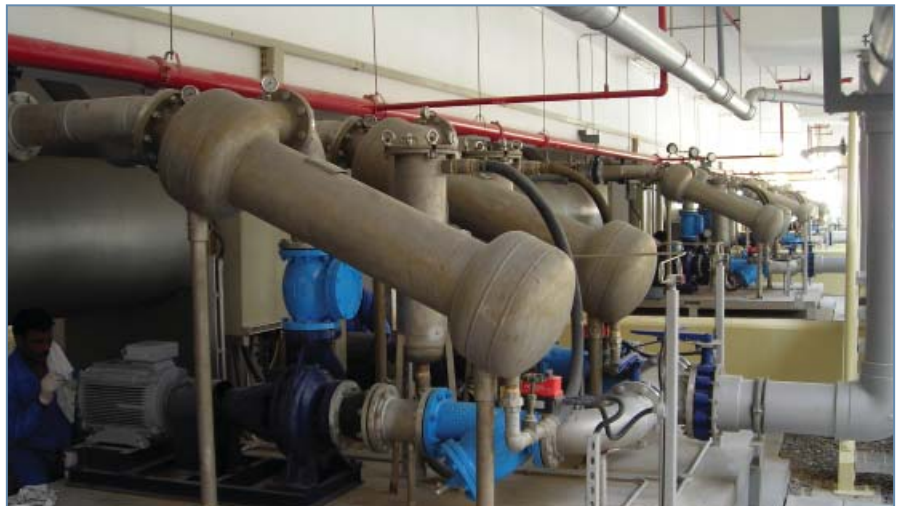
Cooling Tower Filtration and Water Recycling System
