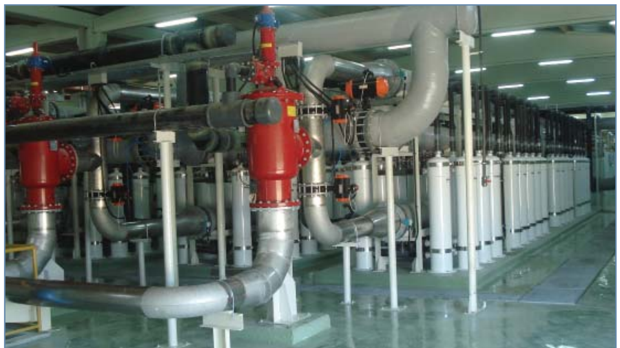
Wastewater Treatment Plant Automatic Filtration prior to UF and RO Systems
