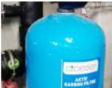
Automated valve filtration systems with FRP tanks
