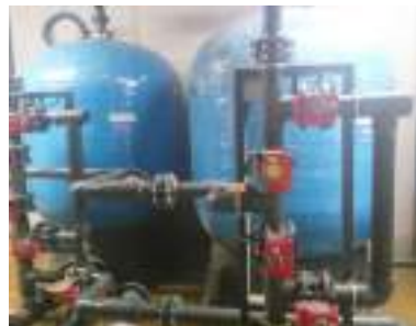
Surface Piped (package piped) filtration systems with Frp tanks
