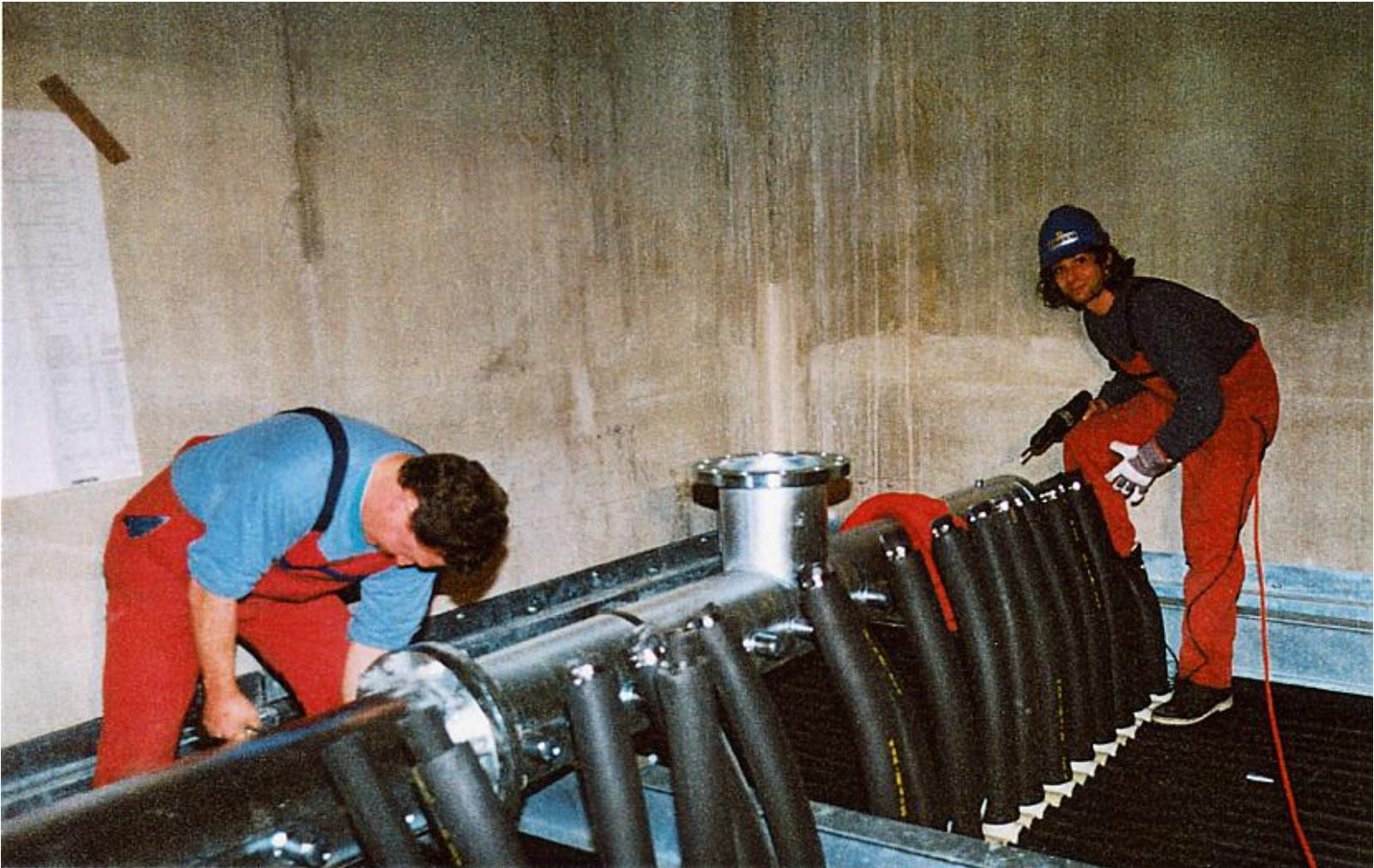
Main header connection to heat exchangers with rubber hoses
