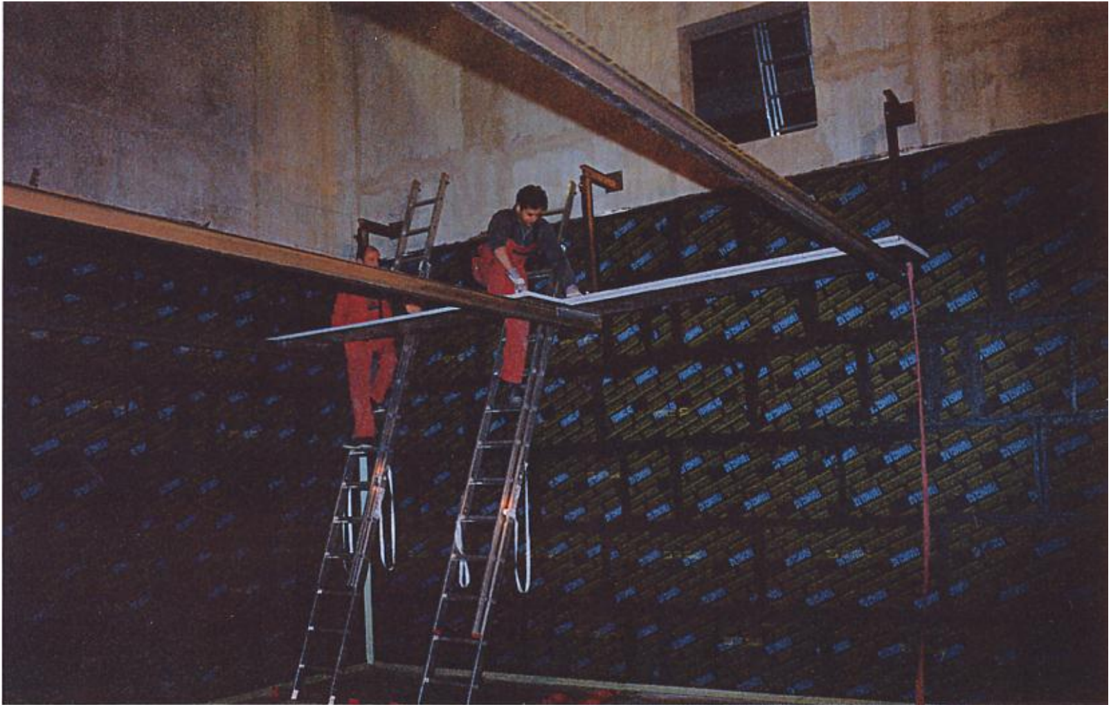
Foamglas insulation of floor and walls
